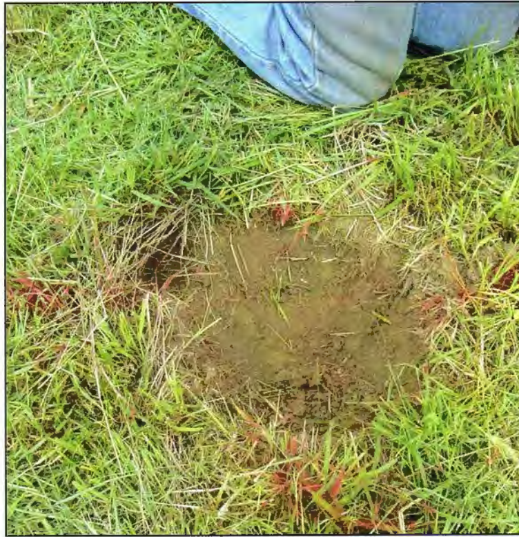
PHOTO 2: Sod removed in conical shape of concrete head.
