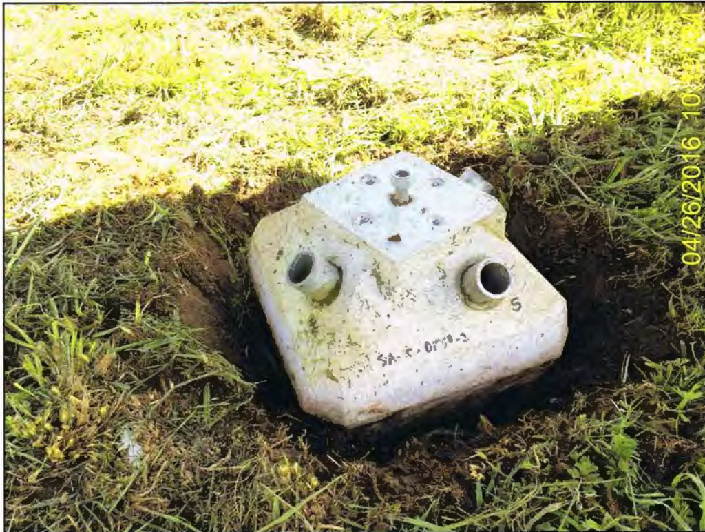
PHOTO 6: Typical Diamond Pier after 1 to 2 inches of soil was removed from around the bottom and sides.
