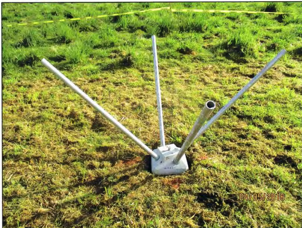
PHOTO 3: Typical concrete head seated and ready for bearing pin installation. Note caution tape in the background to ensure test site was not impacted by vehicular traffic surcharge loads.
